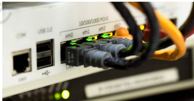
Figure 10.12: Cables connected to a network switch
