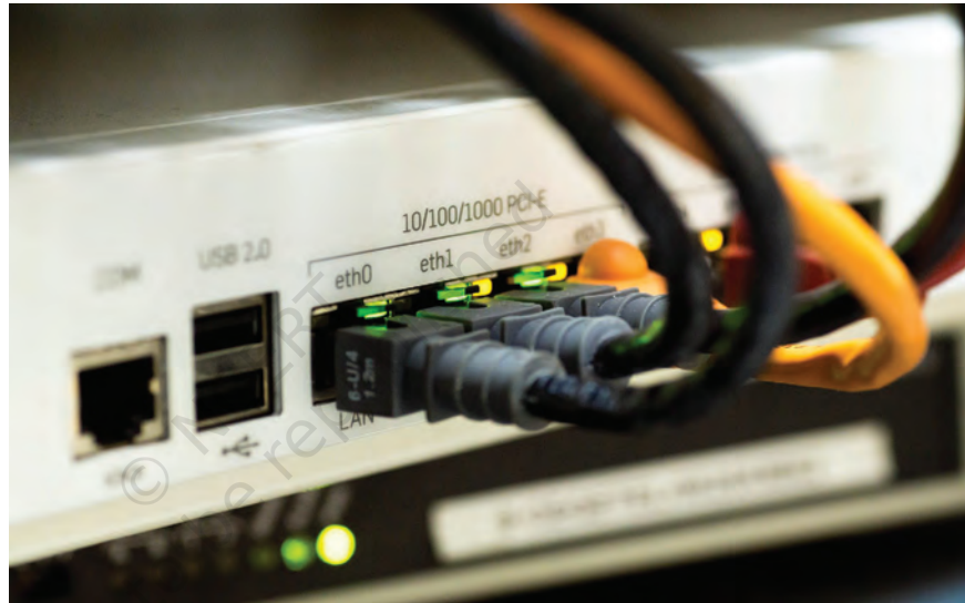
Figure 5.9: Cables connected to a network switch
